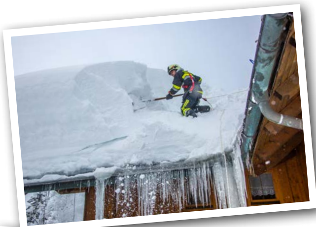
After heavy snowfalls roofs have to be freed from snow to avoid damage.
